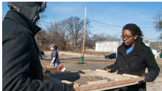
Walnut Hills residents, Matt and Jena Bradley , sifting gravel to grout the pavers.
